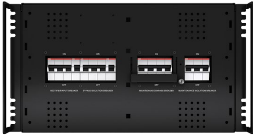
Front view (panel off) offers easy access to breakers
